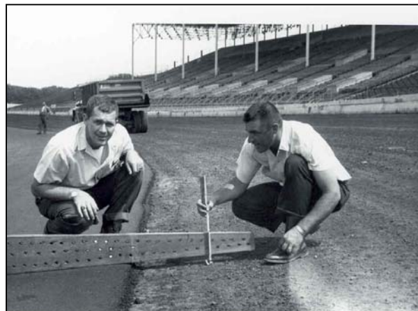
Pictured Left to Right: Dan Ringrose (Project Engineer from Ed Bather & Associates, Inc.) and Lyle Jacoby ensure lift thickness.
