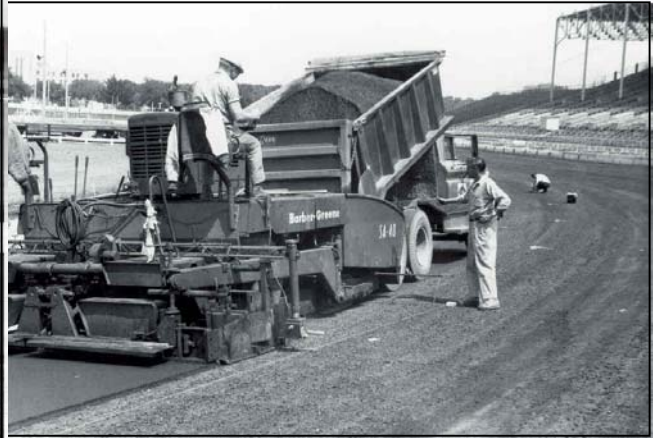
Paving the HMA racetrack in 1964 using an electronic grade control device to ensure proper grade.
