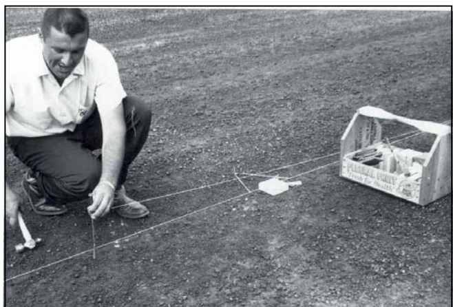
Lyle Jacoby placing the string line on the blocks in 1964. [Lyle is currently Past President (Retired), Pine Bend Paving, Inc. Inver Grove Heights, MN.]
