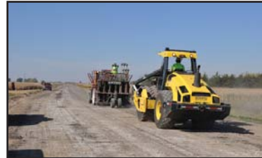
Antigo Construction, Inc. (Antigo, WI) performed the rubblization with a Multi-Head Breaker, followed by a vibratory, Z-bar roller for compaction.
